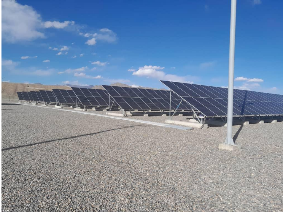
Figure 1a. Solar Power Station in Murghab (3600m above sea level, 700 kWt)
